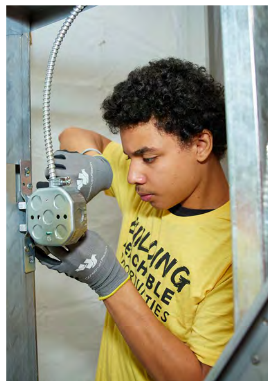
◀ Students in St. Louis learned the proper way to wire and install electrical boxes for wall outlets, switches, and light fixtures to metal studs.
